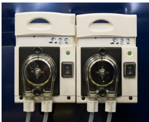
Figure 7: Conditioner and Neutralizer Pumps
