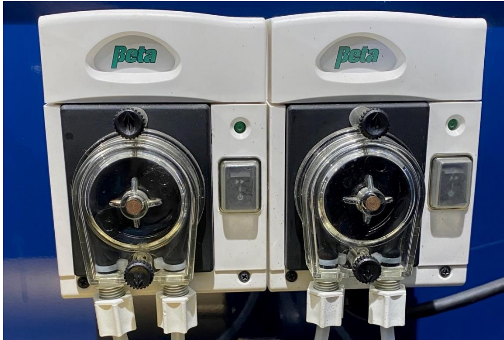
Figure 7: Left: Coil conditioner pump; Right: Neutralizer pump
