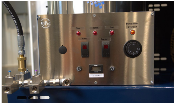
Figure 1: Identification plate location on the right side of the control panel.
