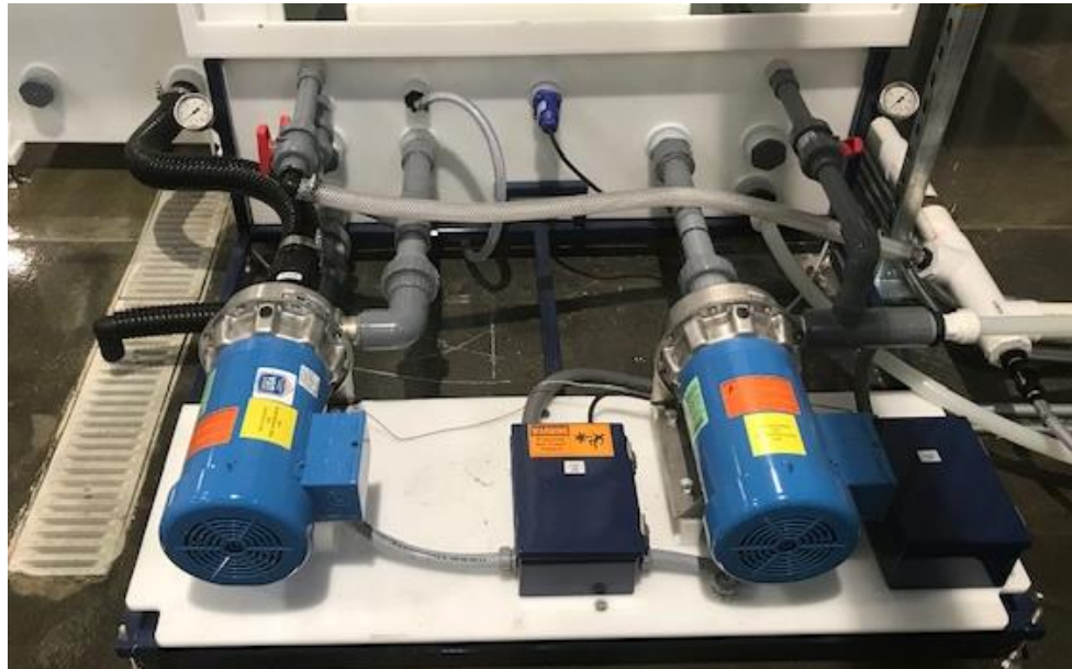
Figure 5: Spray pump (left) and heater (re-circulating) pump (right); note the pressure gauges mounted on the steel frame
