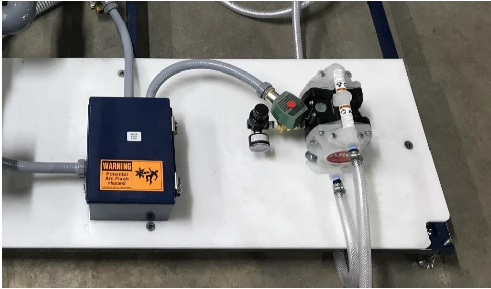
Figure 6: Auto-fill transfer pump
