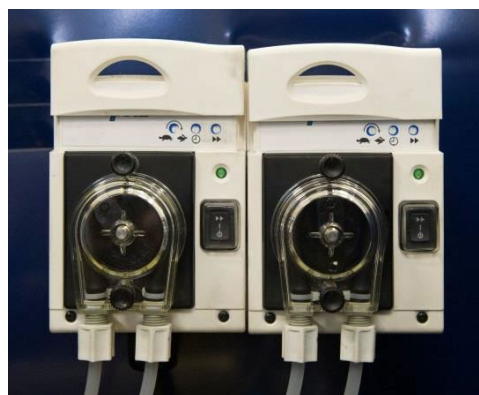
Figure 7: Conditioner and Neutralizer Pumps
