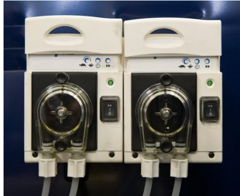
Figure 7: Conditioner and Neutralizer Pumps
